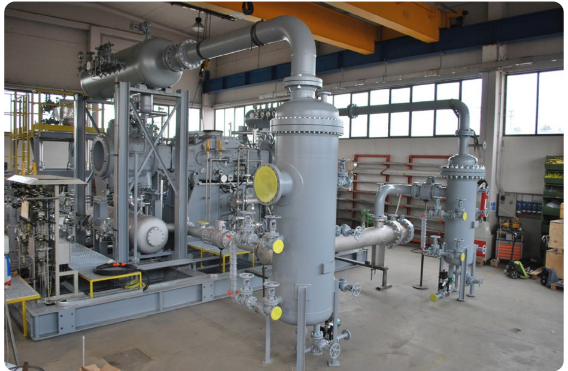
Compressor System with Two-crank horizontal compressor size 190. NEA has offered state of the art solutions for 25 years in Egypt.
